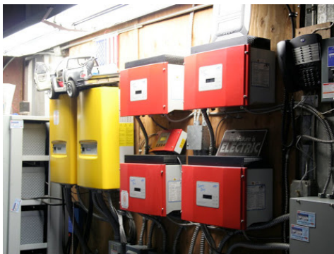
Grid-tie inverters & batteries installed in Strizki's home!
